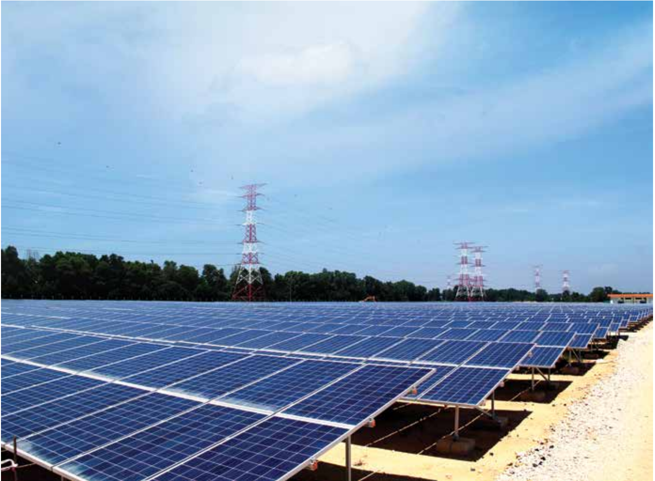
10MW Solar Photovoltaic Farm in Gebeng, Pahang
